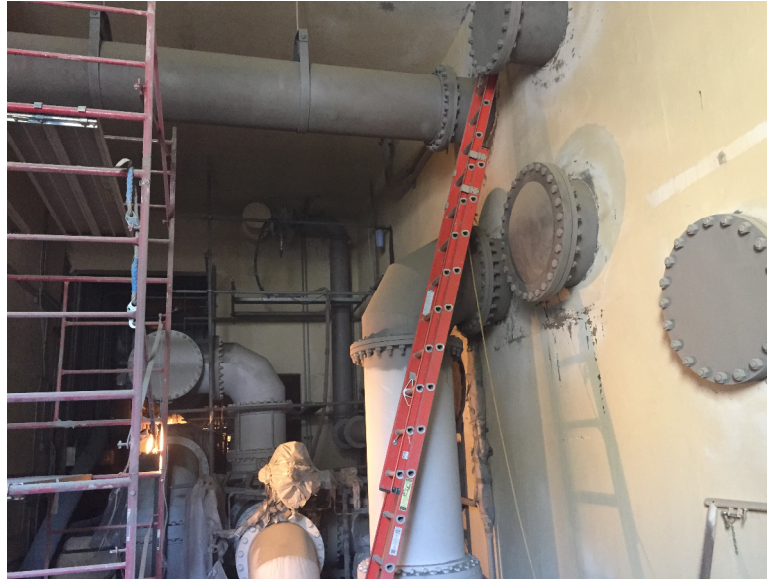
July 1, 2015 – Sandblasting, cleaning and application of prime coat on the filter gallery piping.
