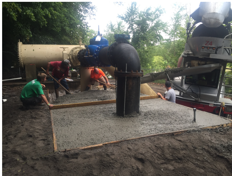
July 9, 2015 – Placing 4000 psi concrete for the new foundation floor slabs of the 2 new buildings at the RAW bypass, schedule 2.
