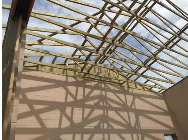
July 20, 2015 – installing the new treated top plates and trusses for the new alum building.
