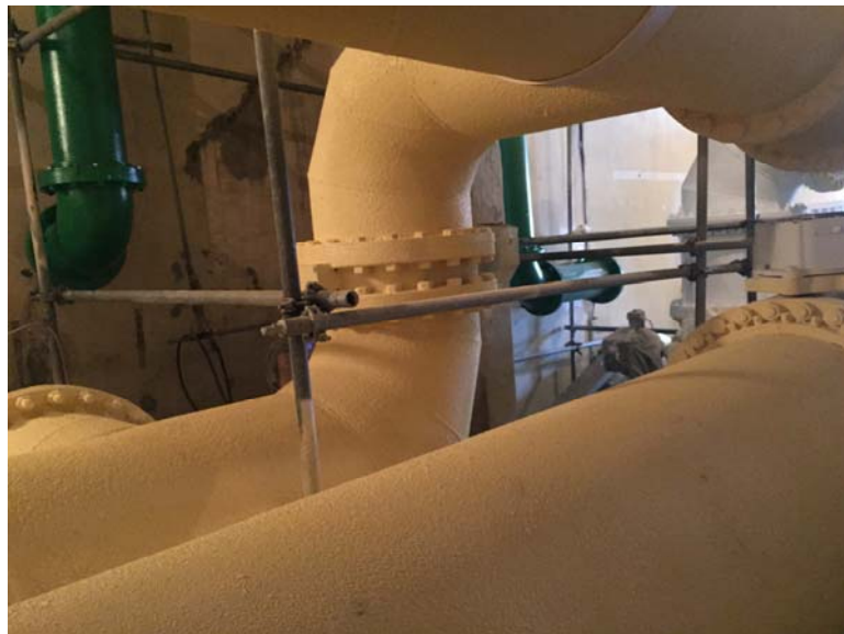
July 21, 2015 –Painting / application of coatings for the piping and walls in the filter piping gallery.
